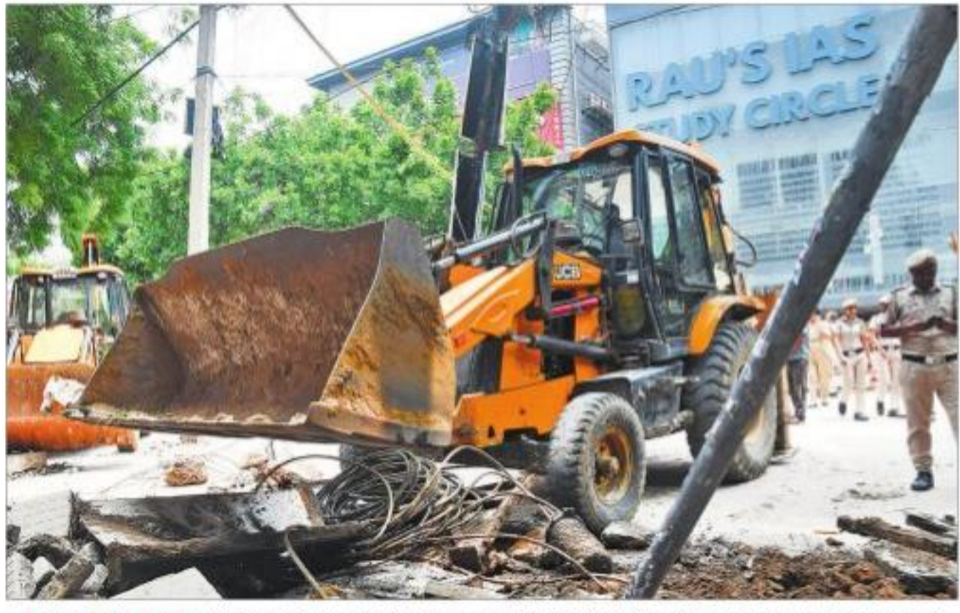
DELHI TRAGEDY: A handful of coaching centres operating in violation of the rules have been sealed, encroachments over drains bulldozed and a high-level probe committee set up. TRIBUNE PHOTO
