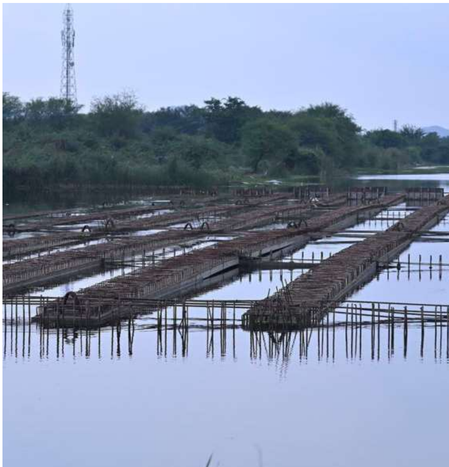
In progress: Ongoing construction of the bridge at Amaravathi, Andhra Pradesh on June 10. RAO G.N.
