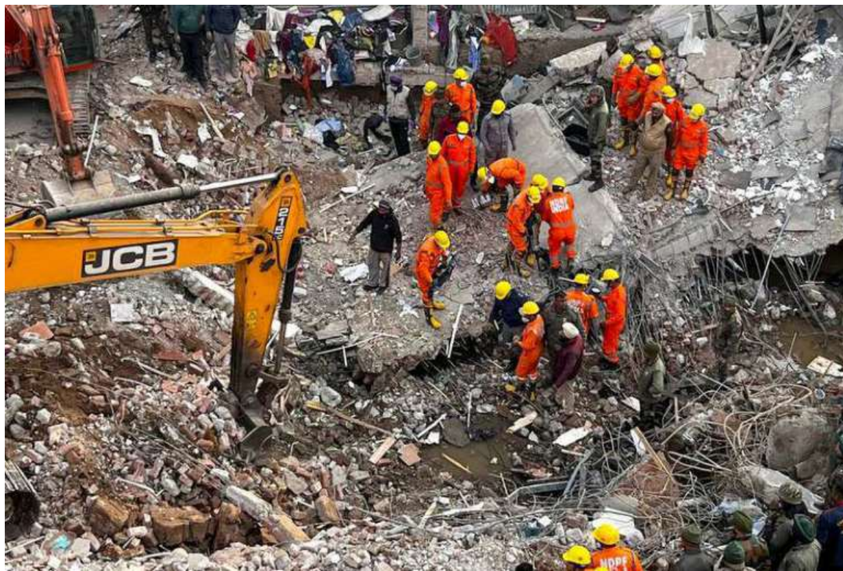
Ground zero: Rescue operations continued on Sunday after a multi-storey building collapsed at Sohana village in Mohali district of Punjab on Saturday evening. Two people were killed in the accident. PTI (REPORT ON PAGE 4)
