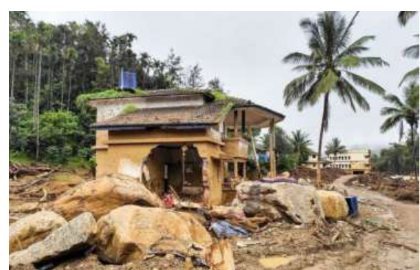
Total havoc: A damaged house and the terrain in the Chooralmala village after the recent landslides. PTI
